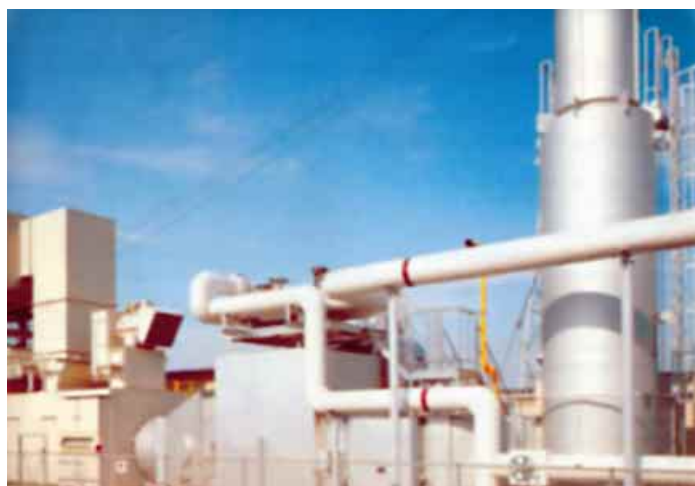
4,000kW gas turbine cogeneration system (Nishio Plant)
