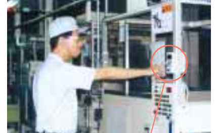
Energy-control equipment (Nishio Plant)
