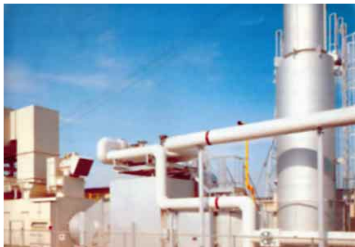
4,000kW gas turbine cogeneration system (Nishio Plant)
