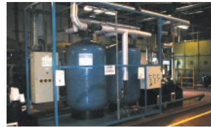
Rainwater collection tanks
