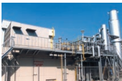
Takatana Plant's 6,500kW cogeneration system, DENSO's eighth facility
