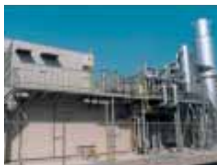
Cogeneration at Takatana Plant
