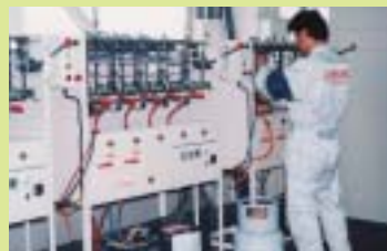
CFC transfer equipment
