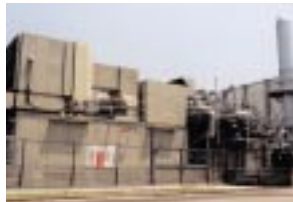
Cogeneration facilities in the East Factory of the Anjo Plant
