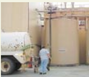
Sludge, collected and stored in the plant, is efficiently processed
